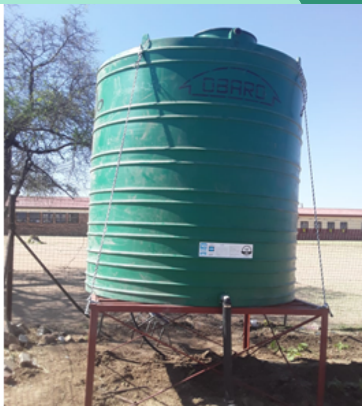
The 5,000-litre water tank installed at the school
